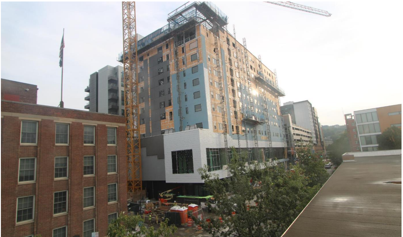
The Asteri affordable housing project under construction in the City of Ithaca. Image credit: Ithaca Downtown Conference Center
