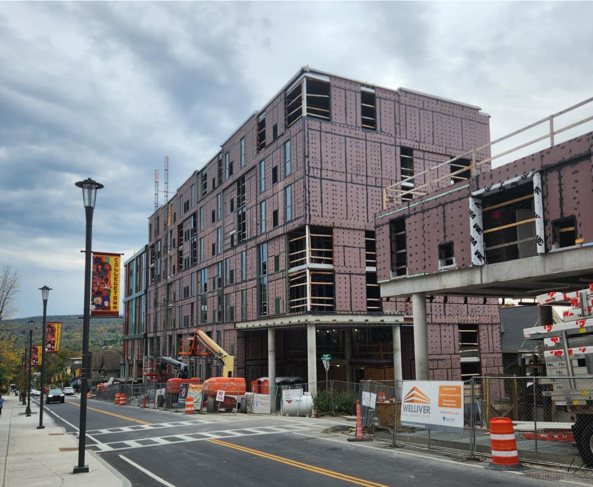
Catherine Commons student housing under construction in the Collegetown neighborhood of the City of Ithaca
