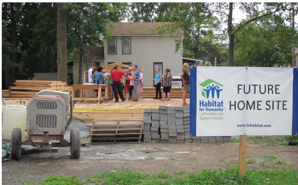
A Habitat for Humanity home under construction in the City of Ithaca.
