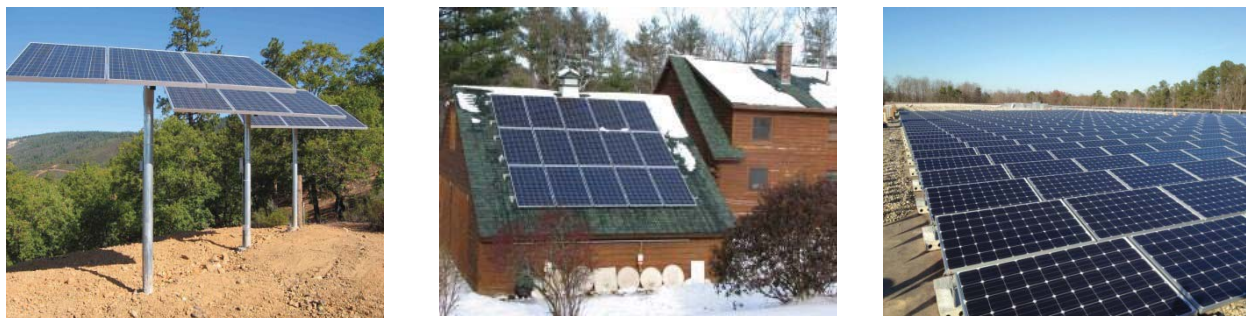
Figure 38 Ground-mounted system, Roof-mounted system and PV Farm
