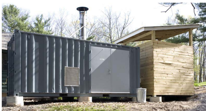
Figure 48 Cayuga Nature Center, in Ithaca, NY, has a 0.5 MMBtu wood chip-fired boiler (housed in a shipping container outdoors) that heats the main building, saving them about $15,000 each year on propane costs
