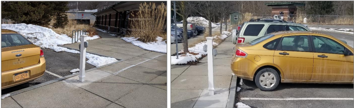
Figure 4: Recycling and Materials Management PEV Charging Infrastructure
