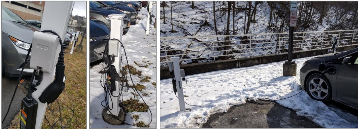
Figure 1: Mental Health Department EV Charging Infrastructure
