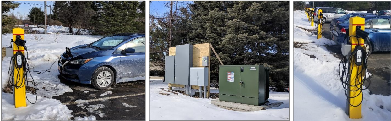
Figure 3: Health Department PEV Charging Infrastructure
