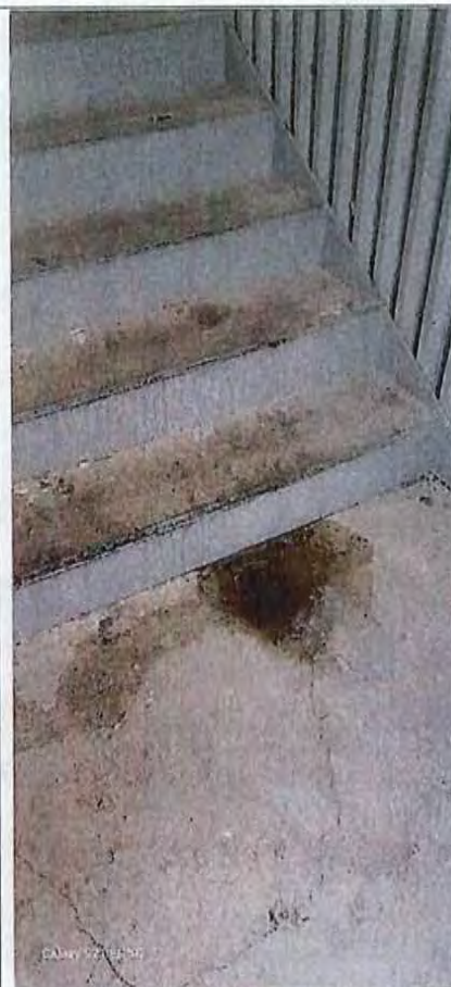
Figure 5b. Urine. Between 7 th and 8 th floors.
