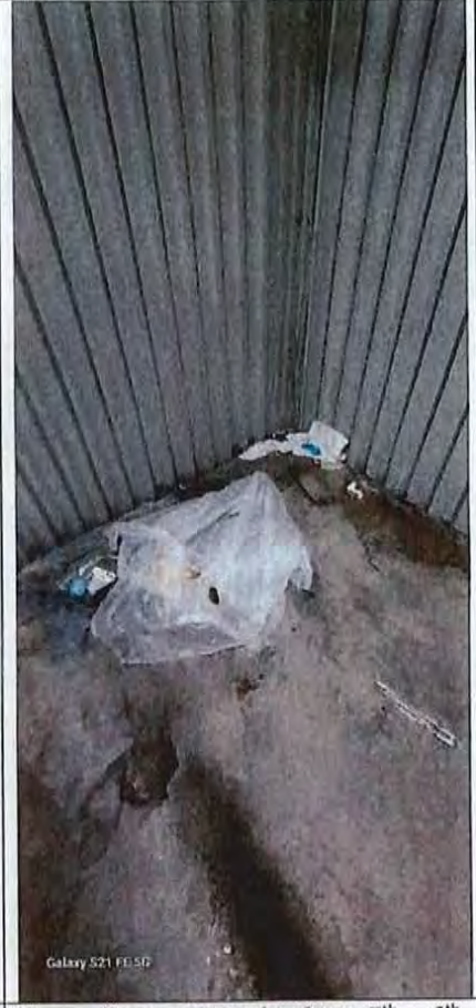
Figure 9c. Feces and refuse. 5 th – 6 th floors – east stairwell.
