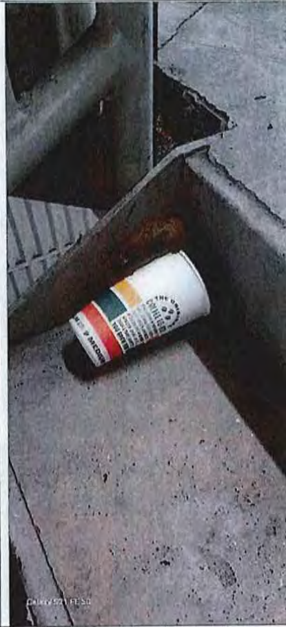
Figure 9b. Feces in disposable cup. 5 th -6 th floors – east stairwell.
