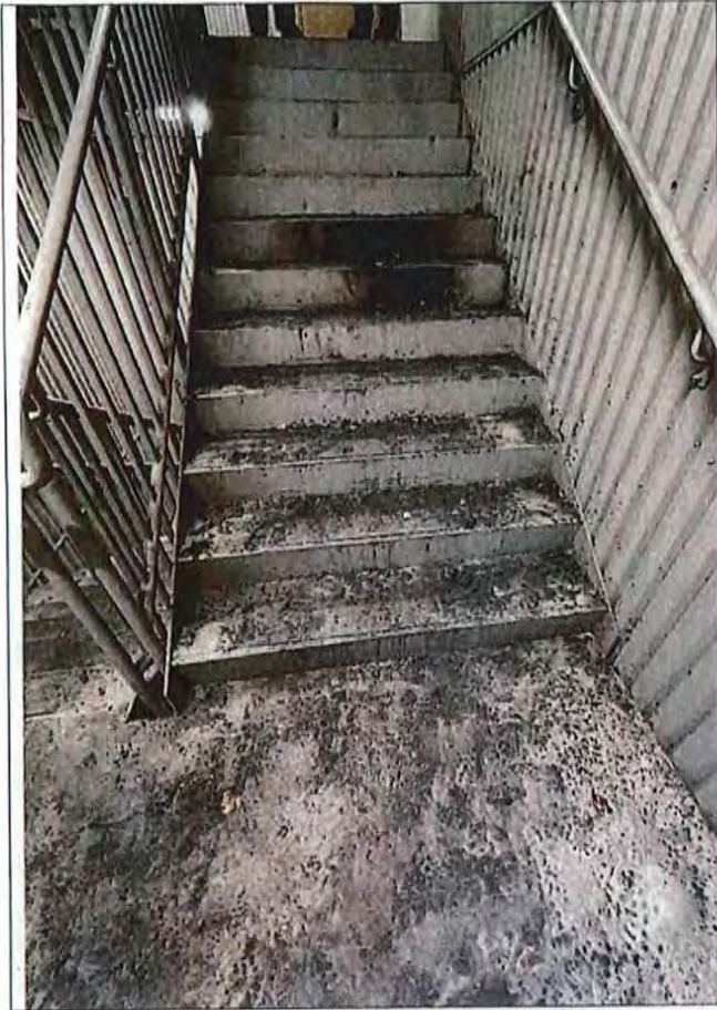
Figure 15a. Soot, ash and debris from fireworks. Note: Reportedly, fireworks were set off over the 1/25 – 1/26 weekend, necessitating the evacuation of the building.
