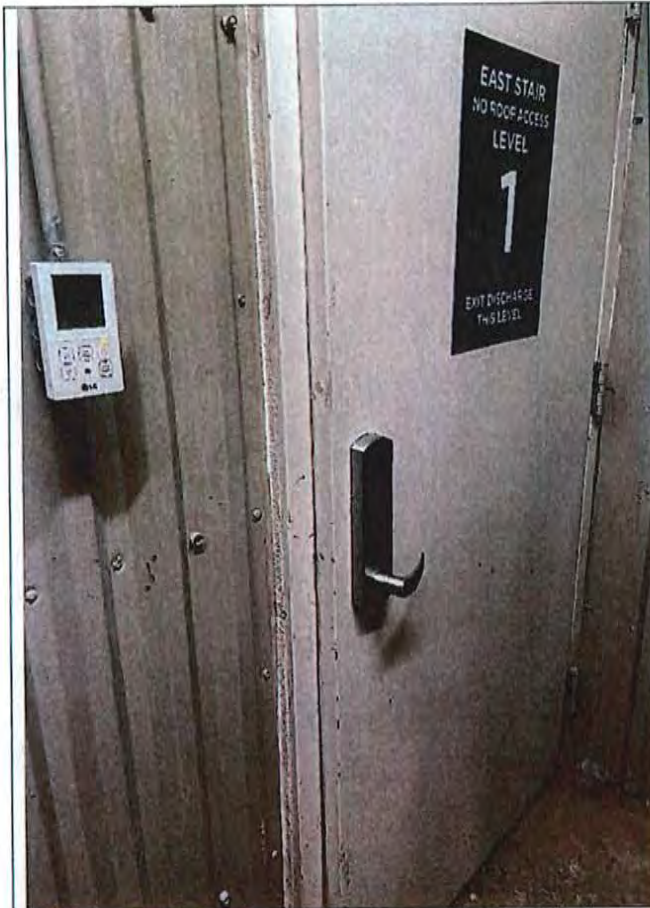
Figure 16a. 1 st floor fire door to east stairwell does not appear to close properly.
