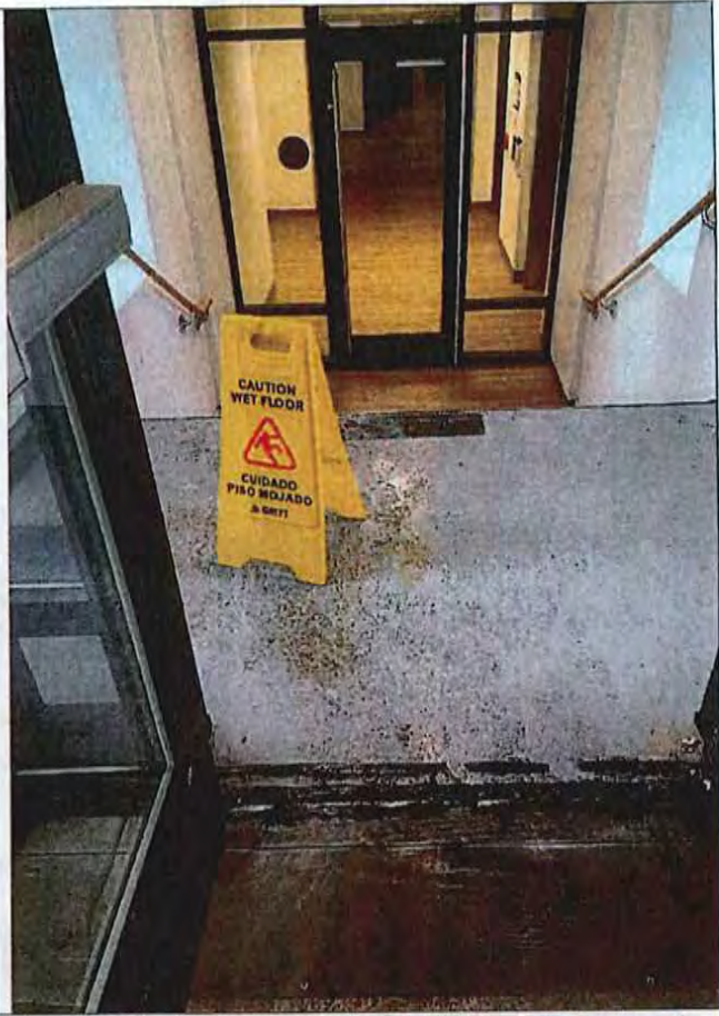
Figure 16b. Frozen urine inside 4 th floor entrance to Asteri Ithaca from Green St parking garage.
