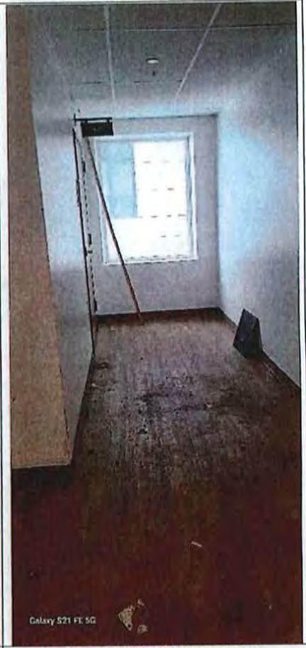
Figure 4c. Outside 6 th floor trash room (door locked).
