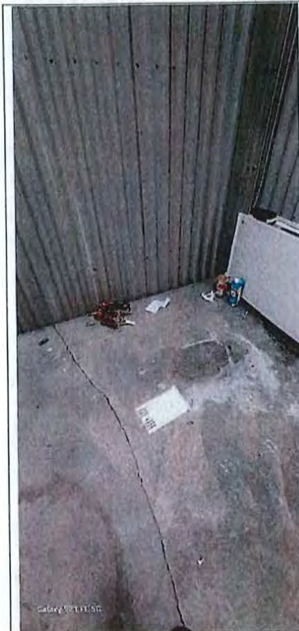
Figure 8a. Spent fireworks remnants and trash. 9 th floor landing – east stairwell.
