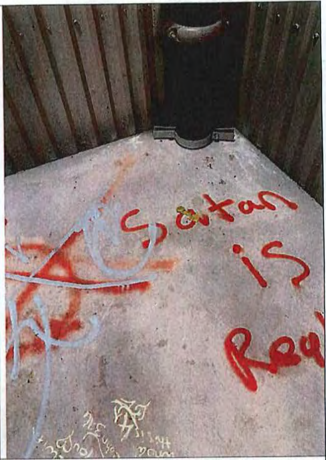
Figure 12b. Used external barrier device contraceptive discarded on landing between 12 th floor and roof access (west stairwell).
