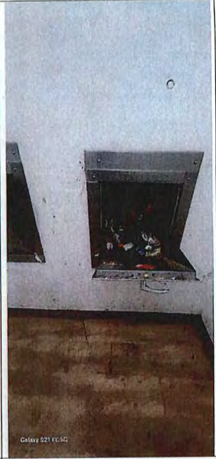
Figure 2c. Chute clogged. Trash room – 4 th floor.
