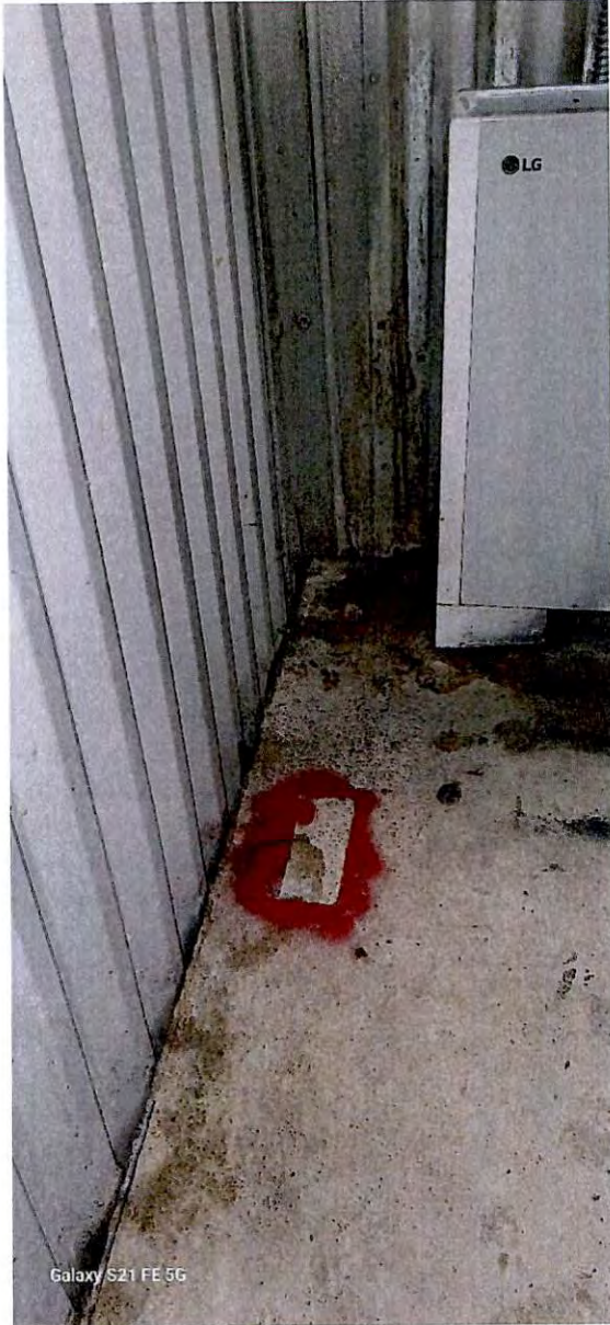
Apparent urine. W stairs, 7 th floor
