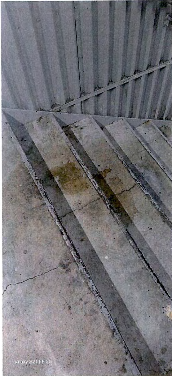
Apparent urine. W stairs, 7 th floor
