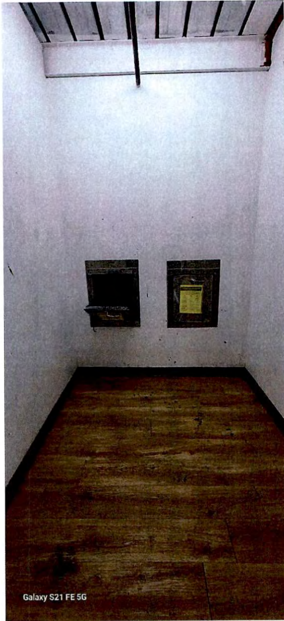
One chute door open. 5 th floor trash room
