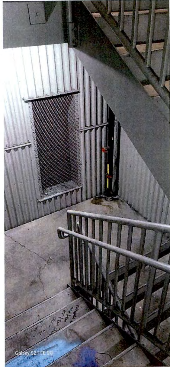
Apparent urine. E stairs, 6 th floor
