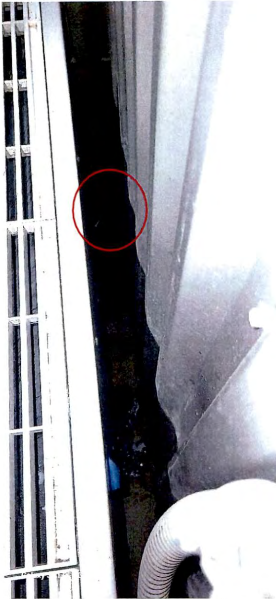
Hypodermic needles behind heating register. W stairs, 2 th floor
