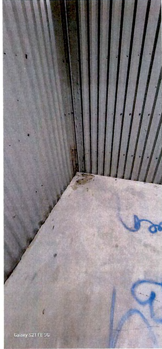
Apparent urine. W stairs, 9 th floor
