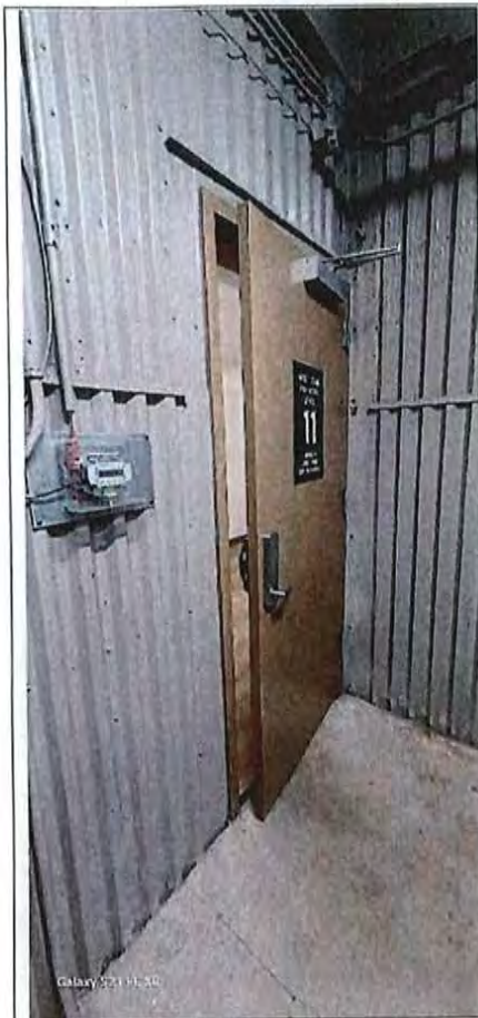
Figure 7a. West stairwell fire door. Self-closing mechanism not functioning properly.
