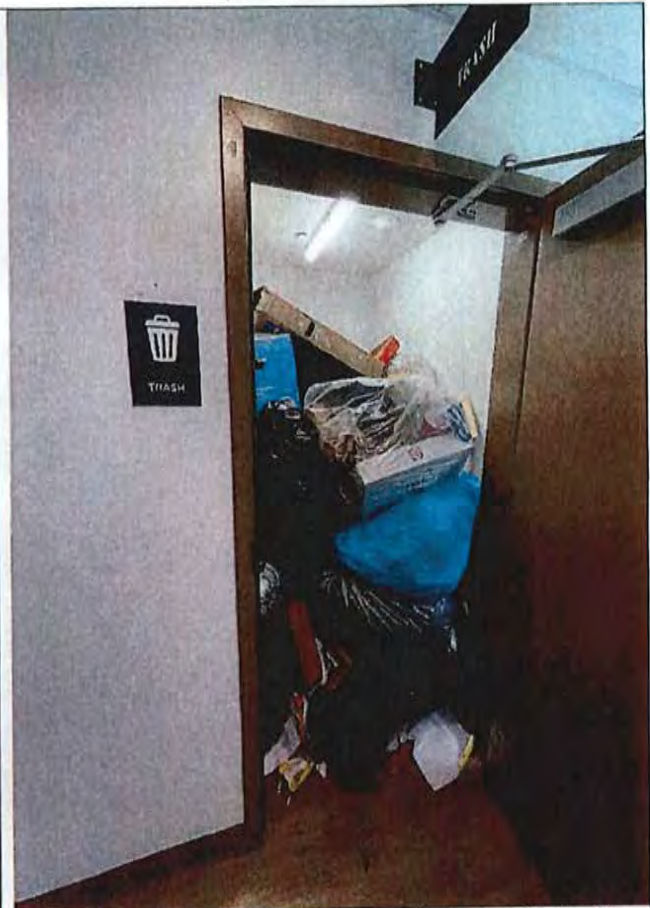
Figure 11b. 12 th floor trash room (room unlocked by temporary, 3 rd party cleaning staff).
