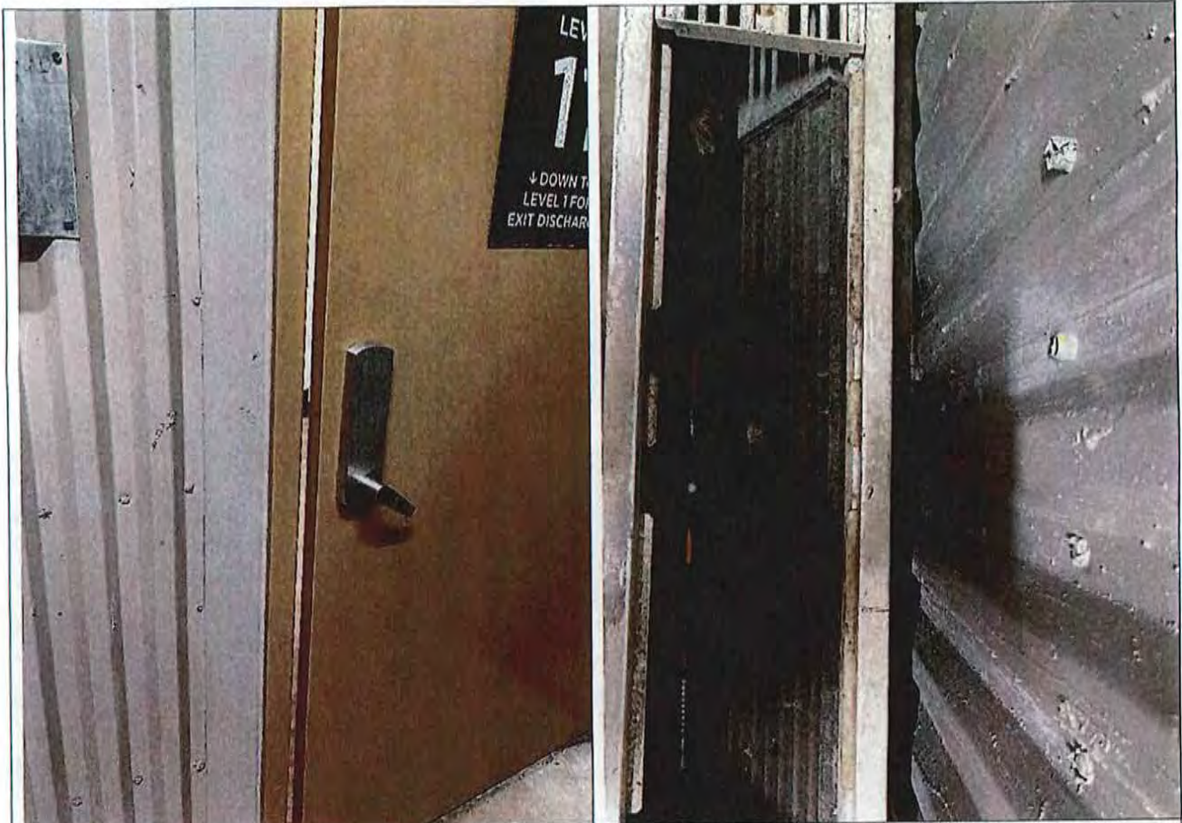
Figure 9a. 11 th floor fire door to west stairwell does not close completely or latch.
