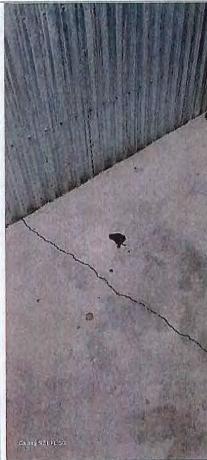
Figure 1b. Dried blood. 3 rd – 4 th floor landing – west stairwell.
