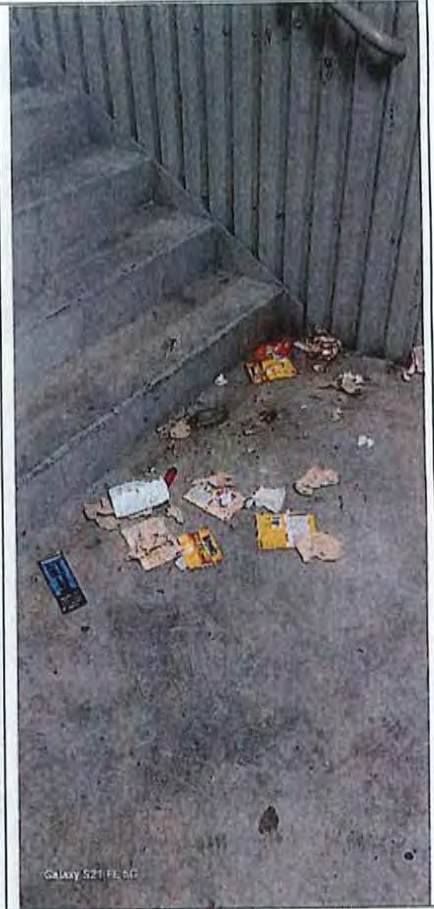
Figure 8c. Refuse. Between 7 th and 8 th floors – east stairwell.
