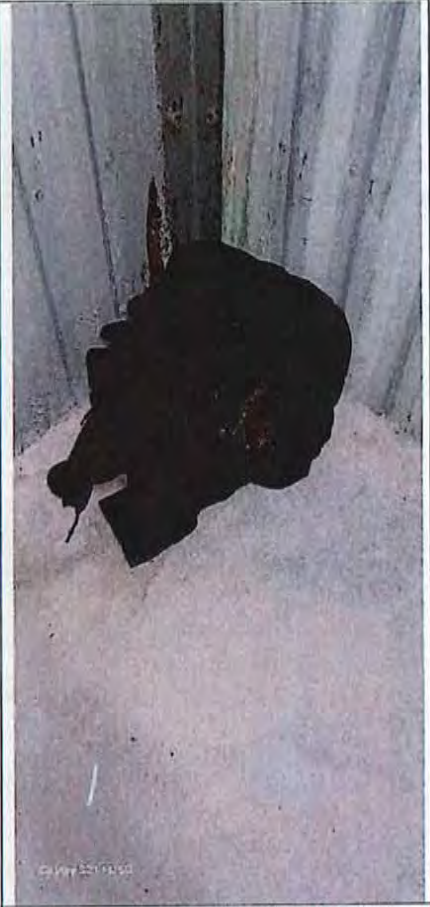
Figure 1c. Feces on wall and jacket. 4 th floor landing – west stairwell.
