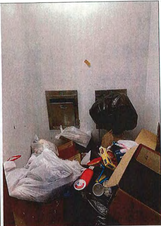
Figure 4b. 7 th floor trash room – chutes open.
