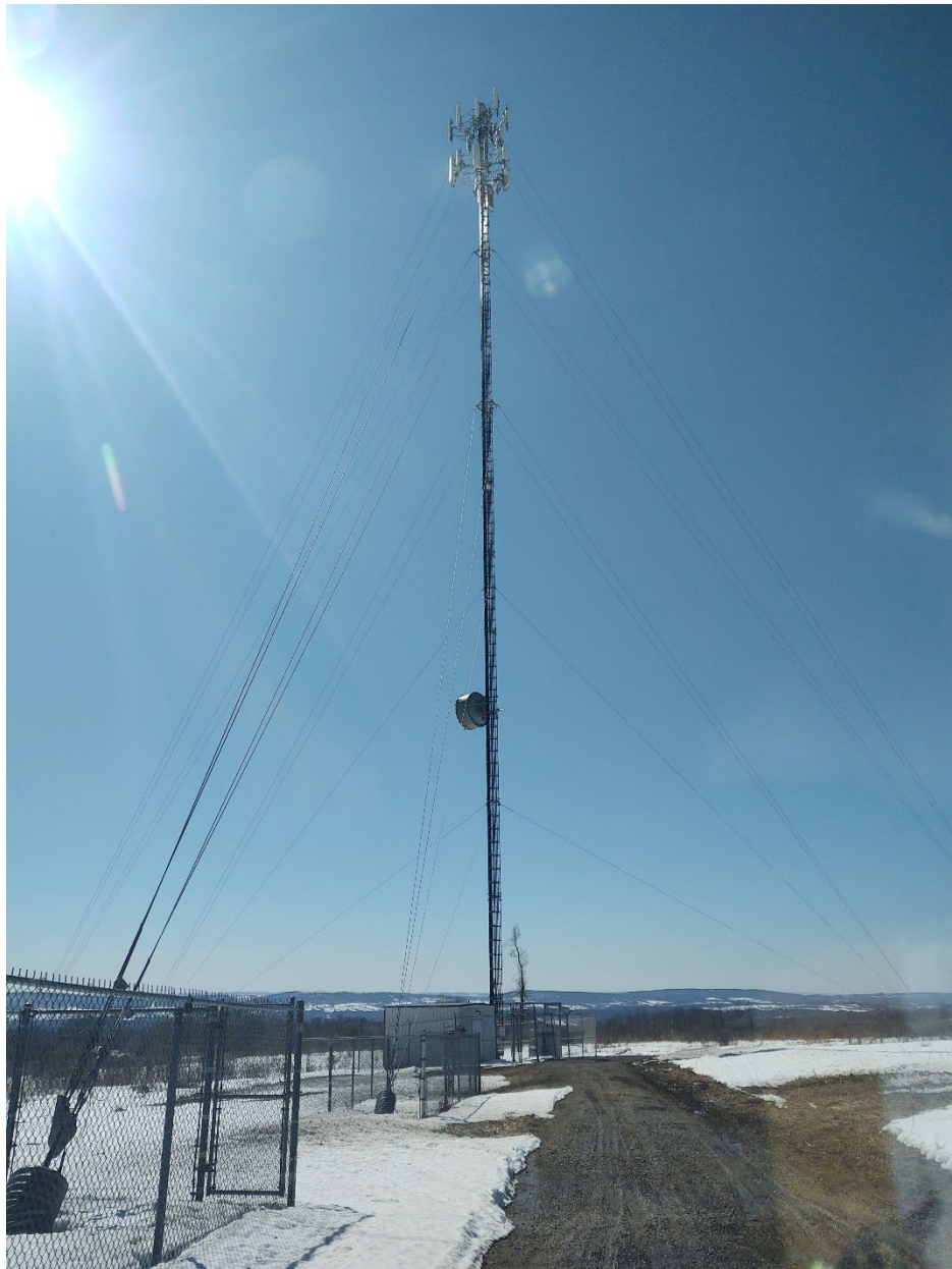
FIGURE 9: GUYED LATTICE POLE TOWER
