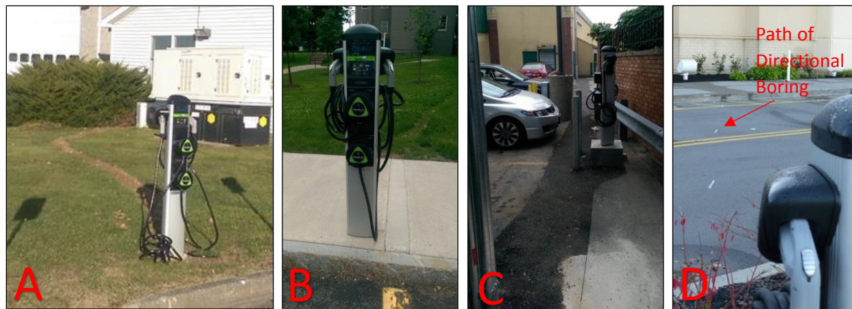
Figure 2. If there is no parking space adjacent to a building where the EV charging station can be wall-mounted, look for locations where the conduit path for power can be through grass (A) or only a small portion of sidewalk (B). It is more expensive to cut and repair pavement (C) or to use directional boring under pavement (D)
