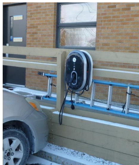
Figure 3. Mounting this Level 2 station on an existing structure helped keep the installation costs low for the Sciencenter
