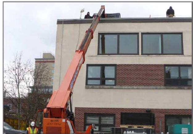
Solar PV installation on Tompkins County Building C, Fall 2012.
