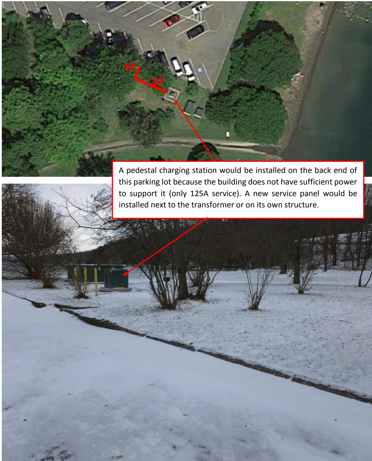
Figure 49. Electrical equipment and conduit run for the proposed placement of a new charging station at Taughanock Falls State Park
