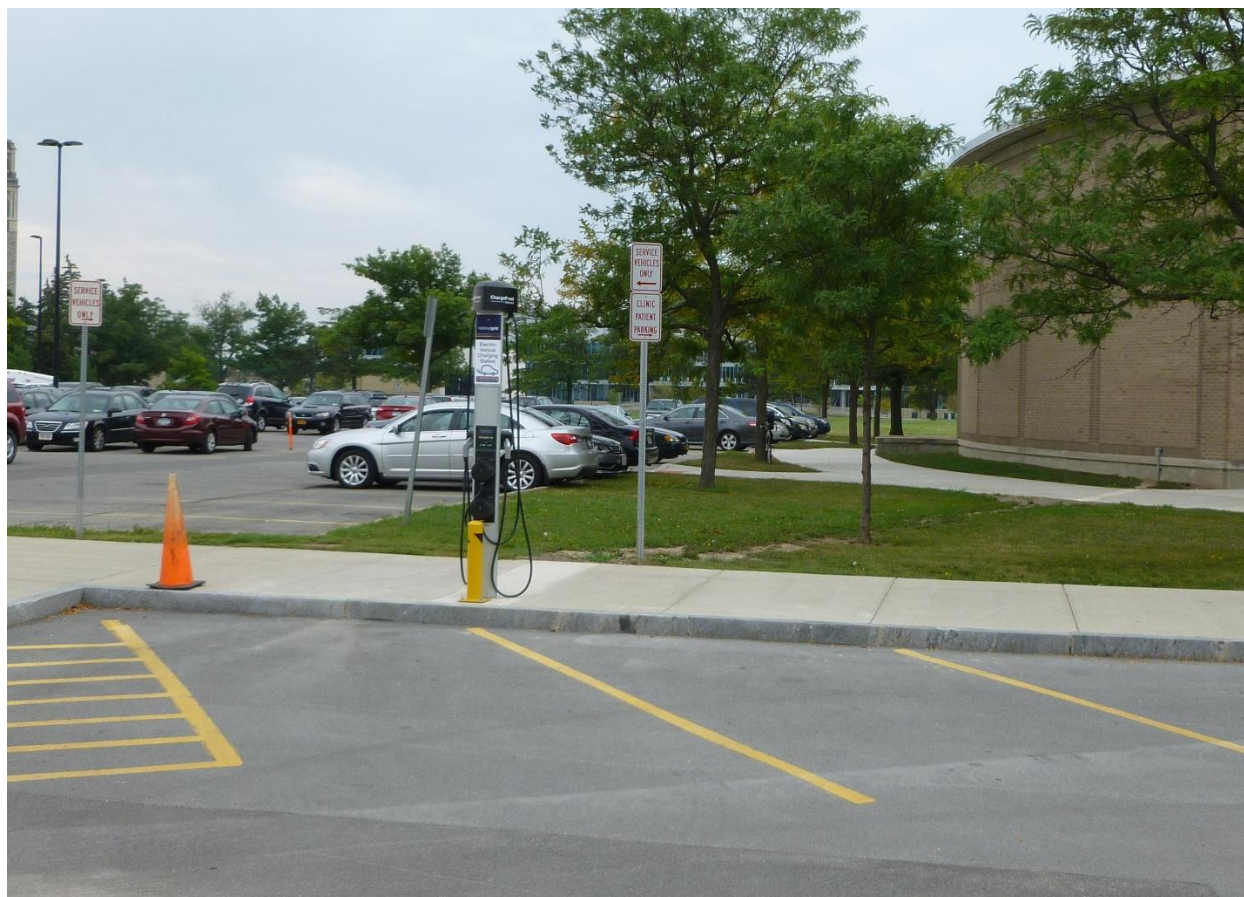
Figure 40. Charging station installation at the University of Buffalo
