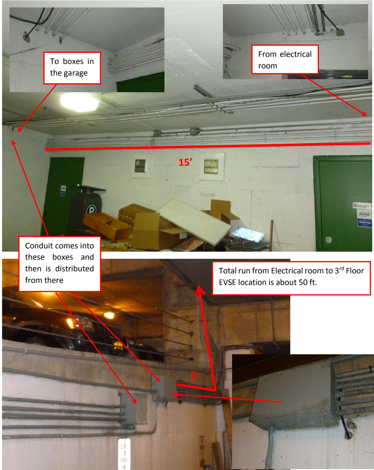
Figure 31. Electrical wiring run for the proposed location for a new charging station at Seneca Street Garage
