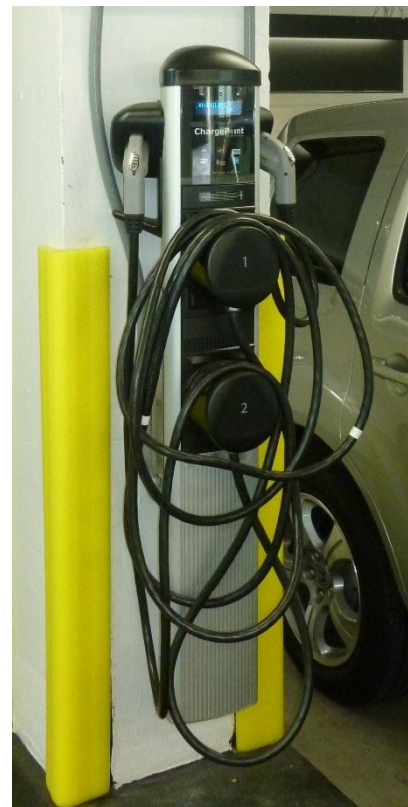
Figure 28. Charging station mounted on a structural column at a rental property in New York City
