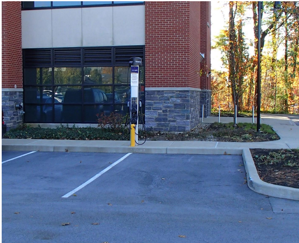
Figure 37. Charging station installed at the Empire State College for Distance Learning
