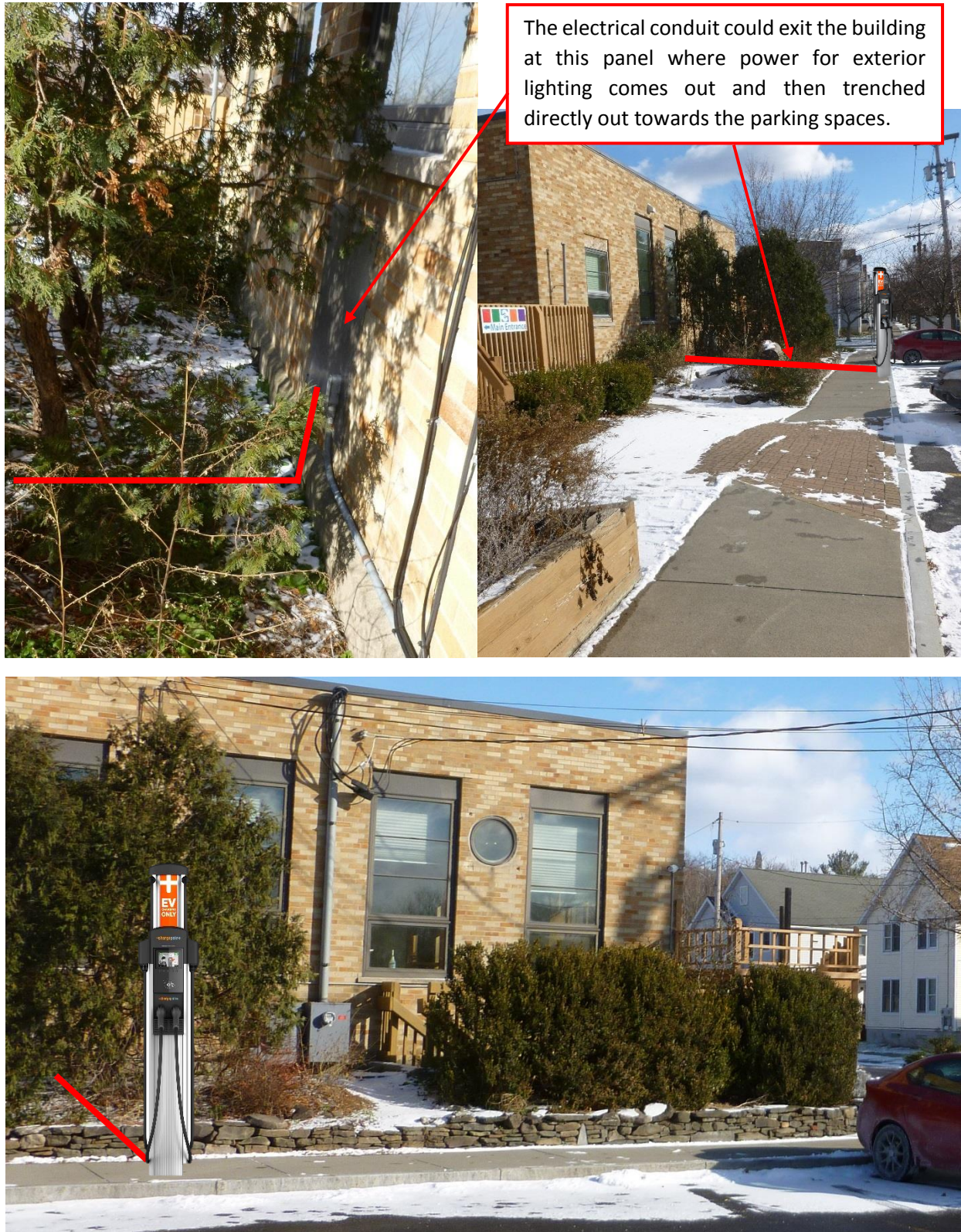
Figure 36. Electrical wiring run for the proposed placement of a new charging station at the Sciencenter
