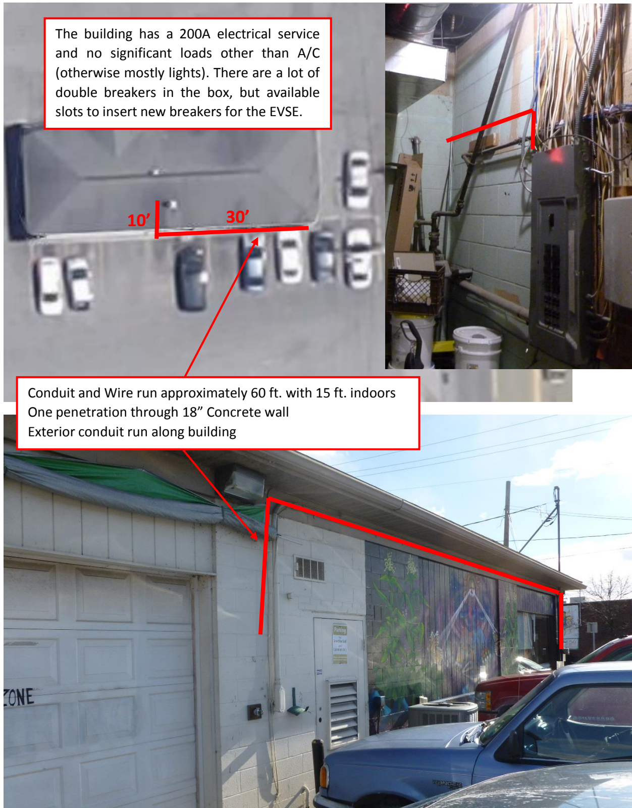
Figure 46. Electrical room and wiring run for the proposed placement of a new charging station at GreenStar
