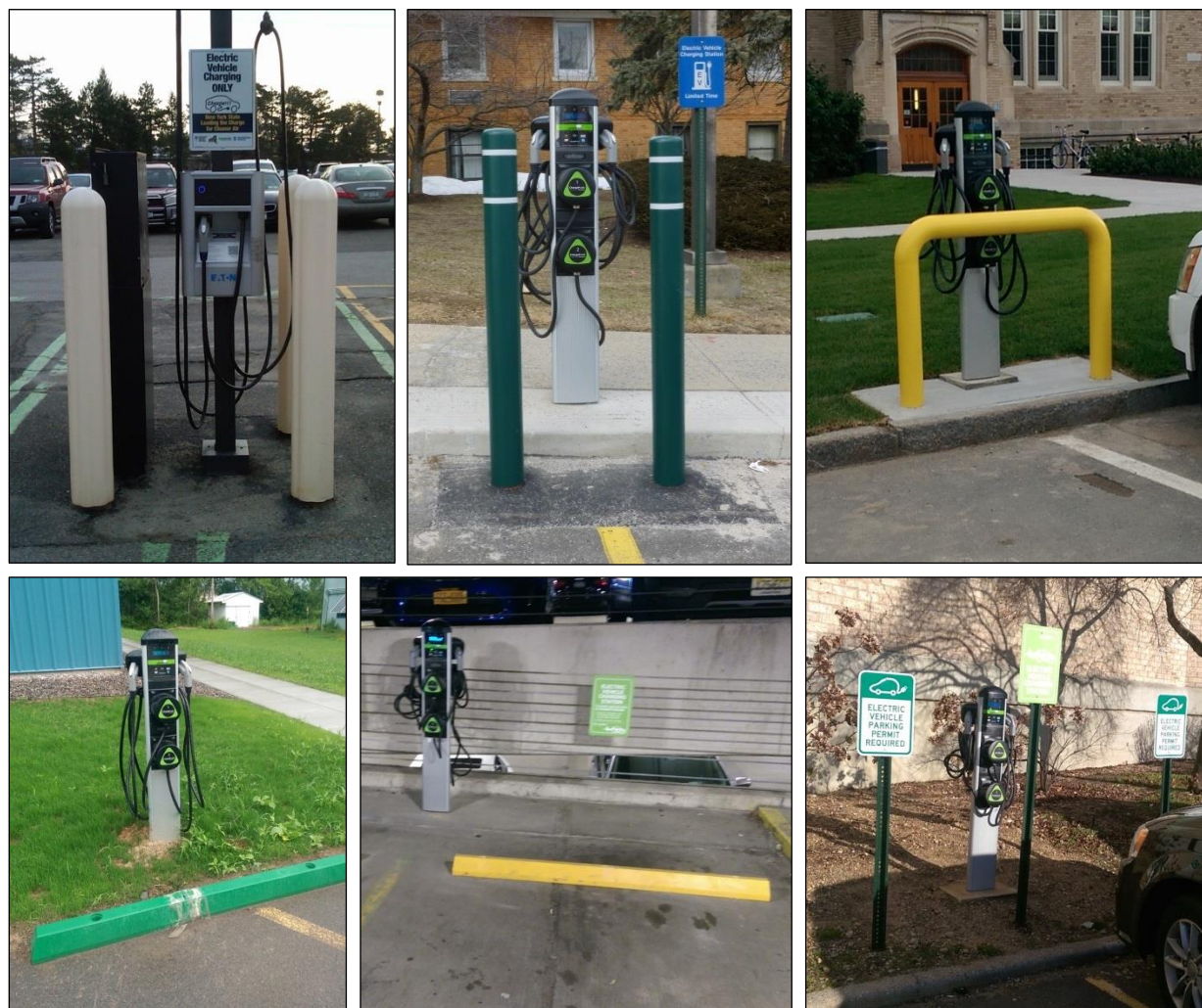
Figure 7: Bollards, tire stops, and sign posts used for charging station protection
