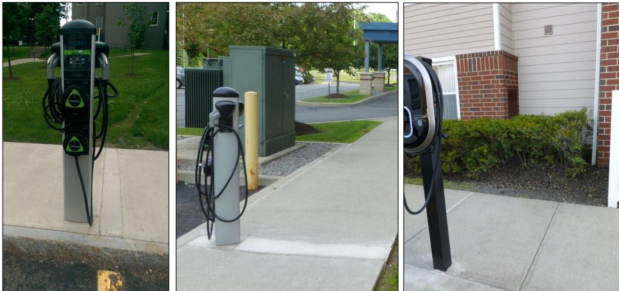
Figure 20: Concrete walkway examples of cut/repair (left and center) and tunneling under (right)
