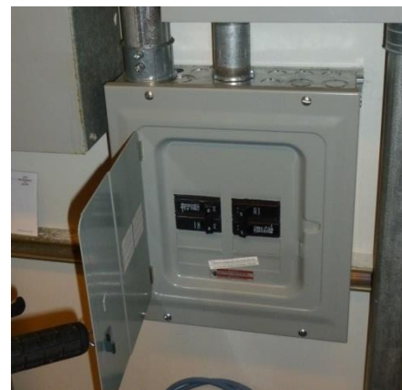
Figure 15: Added subpanel for charging station circuits
