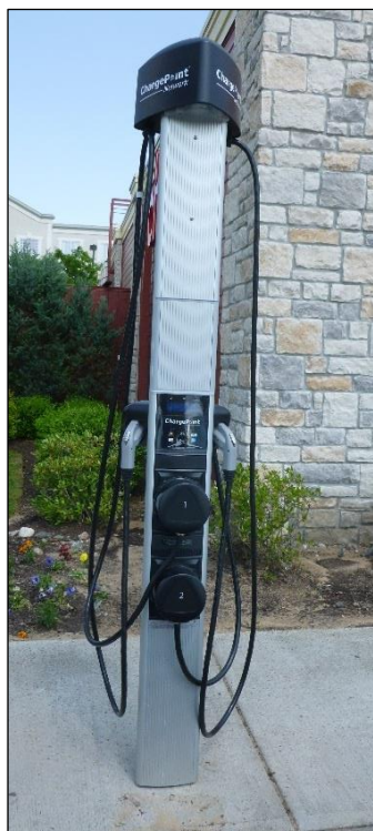
Figure 4: EV charging station with cord management
