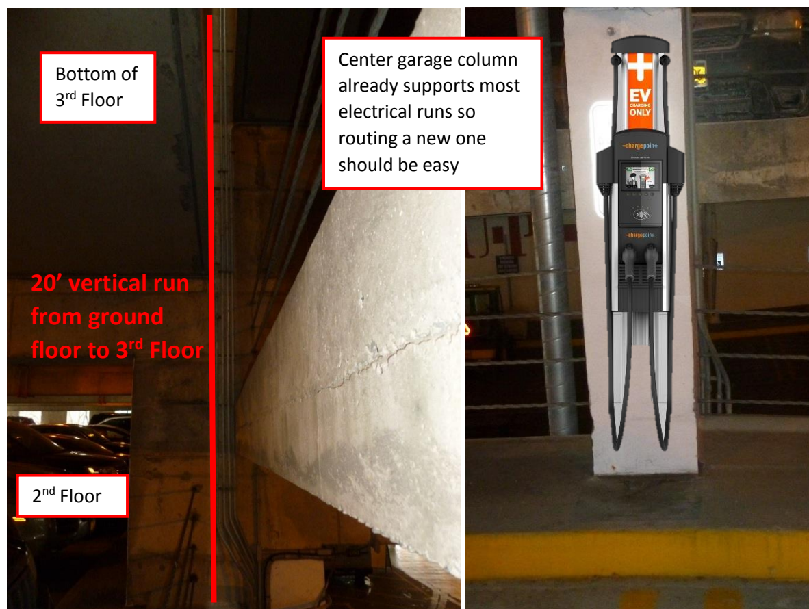
Figure 29. Proposed 3 rd floor location for a charging station at the Seneca Street Parking Garage
