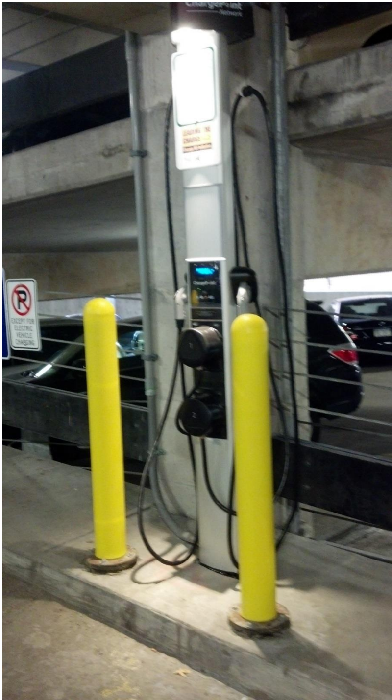
Figure 32. Charging station installed in a City of Rochester Garage
